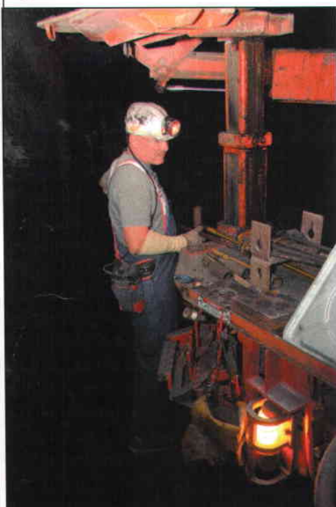
Pat Smillie switches from drill bit to roof bolt at the Prairie Eagle mine.
