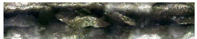
Figure 11. Void as observed from bore-scope video.
