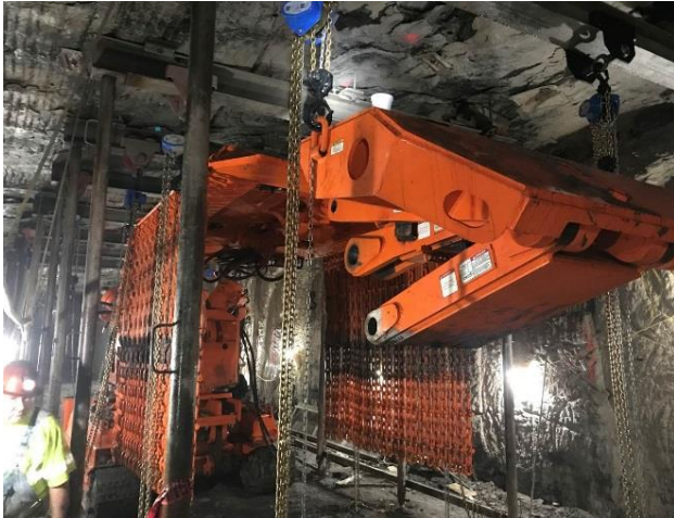
Figure 5. Suspending Roof Support Plate, Chain Side Curtains, Caving Shield and Lemniscate linkages.
