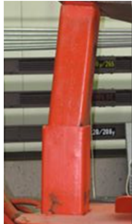
Example of Non-OEM canopy support post, leaning
