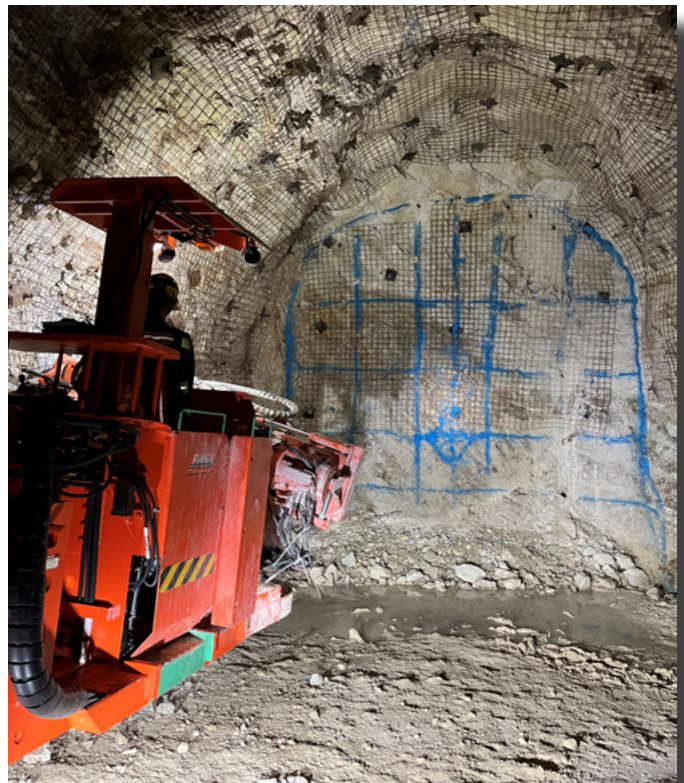
The blue paint grid [pictured above] indicates a drilling pattern on the mine face. During this project at San Xavier Underground Mine, the Cannon jumbo will drill holes into this pattern, then instrumentation will be installed to analyze the impact of blasts propagating in strata. Once the blasting is complete, they will remove the material, re-support the ground in rock bolts, and repeat the process.
