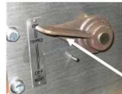
CHECK BREAKER HANDLE FOR PROPER OPERATION
